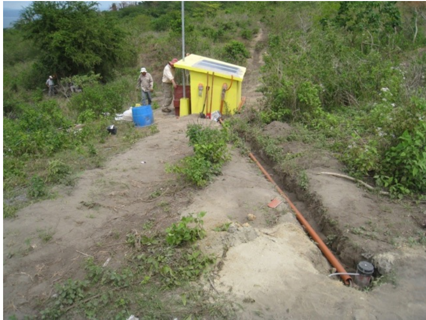
Figure 2. Installation of a continuous resistivity meter in a Shlumberger configuration (CNRS, France) and one borehole tiltmeter (USGS, US) during March 2013 campaign.
